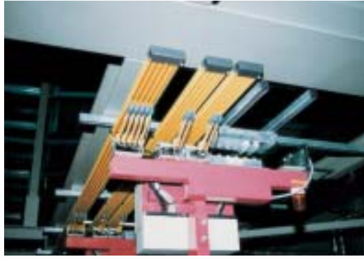
13 pole multipole conductor rail in 33 package distribution centres of the postal service (Post AG)
